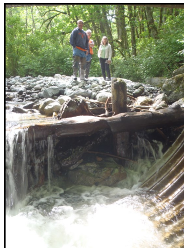
Example of undersized culvert trapping debris and blocking fish passage while potentially increasing flooding upstream.
